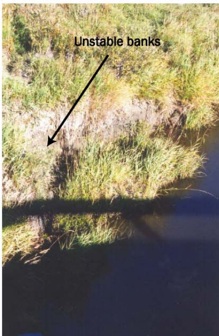
Plate 20. Grasses downstream of road are helping to reduced erosion, but rooting systems are not deep enough to completely eliminate slumping caused by soil saturation. Ideally, the riparian community would be composed of a community of both shrubs and grasses (September 17/2002).
