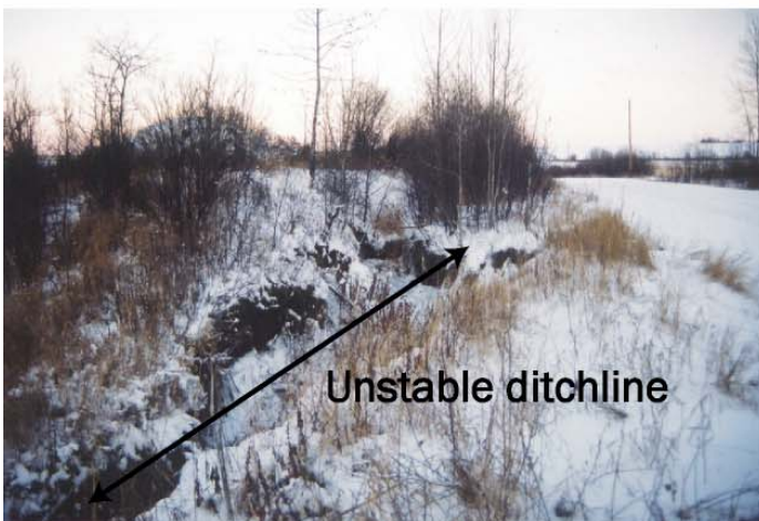
Plate 71. Ditchline is unstable on downstream side of road (resulting from poor drainage and soil saturation (November 12/2002).
