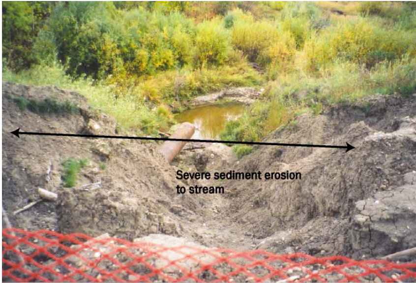
Plate 67. Channel downstream of road showing extensive and severe erosion. Note that the water downstream of the culvert outlet appears to have high turbidity; evidence of sediment transport (September 20/2002).
