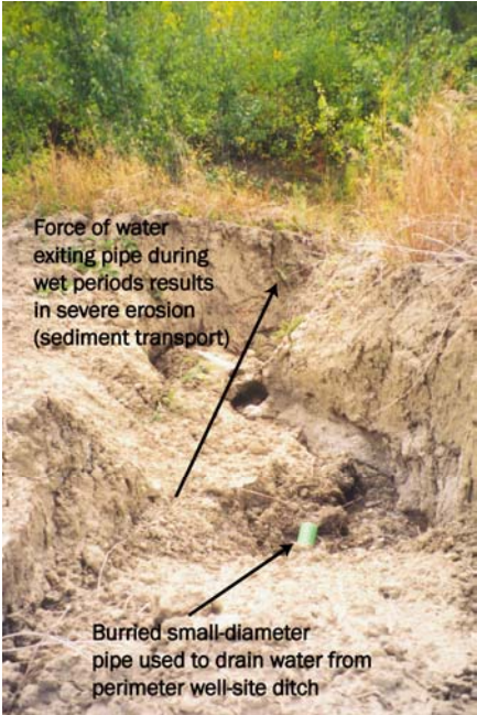
Plate 12. Small-diameter pipe used to drain water collection ditch on oil and gas wellhead site. Note extensive erosion down-slope of pipe resulting from the force of water through the pipe.
