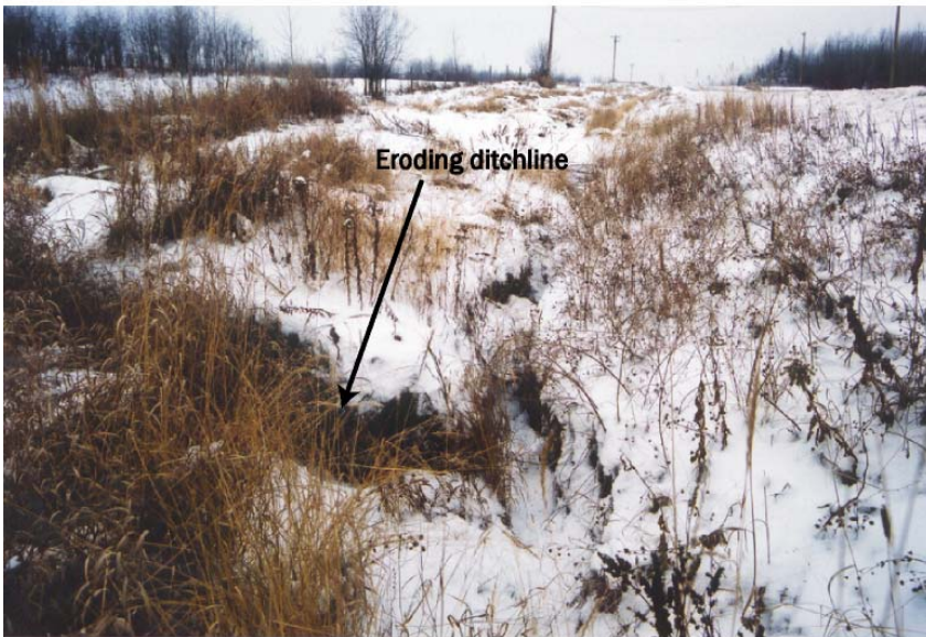
Plate 38. Ditchline on both upstream and downstream sides of the road are susceptible to saturation and slumping (poorly drained) (November 12/2002).
