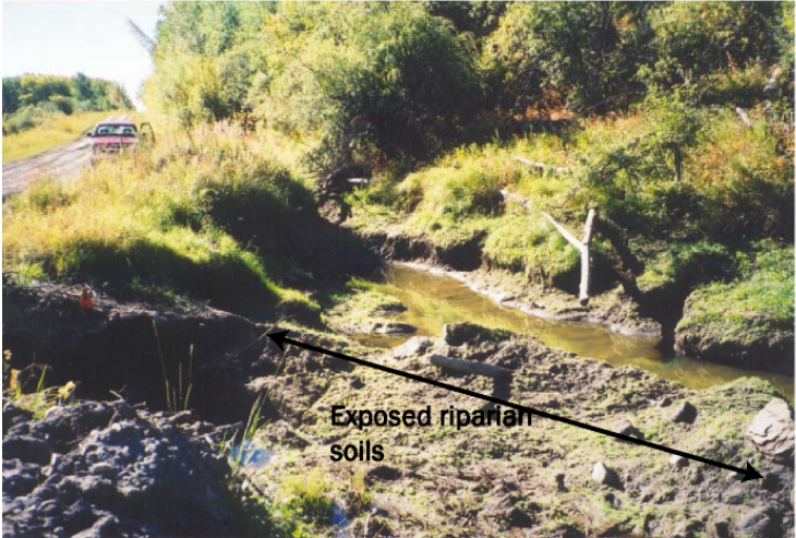
Plate 46. Saturated and exposed soils downstream of road are highly erodable and contribute sediment loads to stream (September 17/2002).
