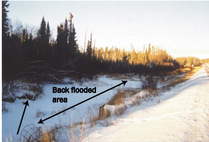
Plate 1. Substantial back flooding upstream of road (channel approaches road from a steep angle). This backflooding resulting from poor drainage is resulting in soil saturation and slumping (November 11/2002).
