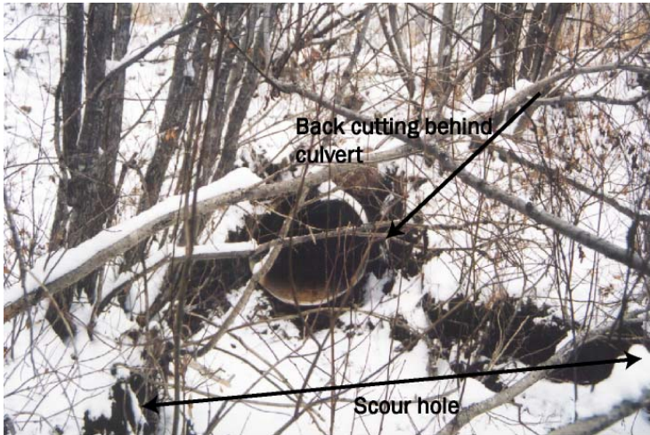
Plate 82. View of culvert outlet downstream of road. Note that there is a substantial scour hole and undercutting behind the culvert (November 12/2002).
