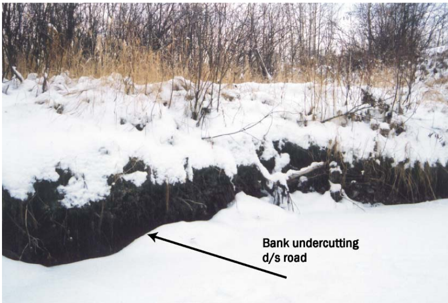
Plate 16. Bank undercutting in scour hole immediately downstream of culvert (November 11/2002).
