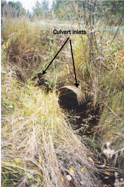
Plate 77. Culvert inlets upstream of road. Note that riparian shrubs and grasses are providing stability to soils (very little exposed soil) (September 19/2002).
