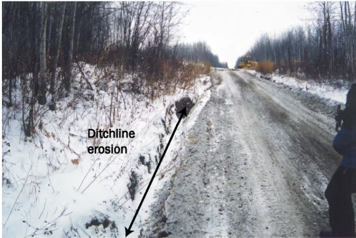
Plate 83. Severely eroding ditchline upslope of channel. The ditchlines on both sides of the road are contributing sediment loads to the stream (November 12/2002).
