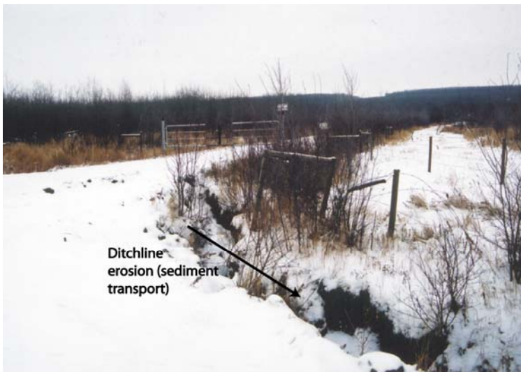
Plate 15. Ditchline erosion observed on private oil and gas road. Ditchline erosion is a common occurrence in the Charlie Lake watershed, particularly where there is any sort of slope (fine sediment is highly erodable, and likely contributes to stream channel sediment loads).
