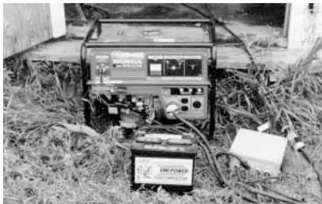
Figure 7. Automated gas powered generator system
