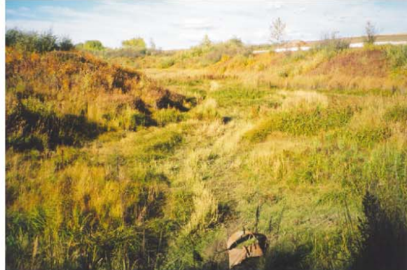
Plate 40. View upstream of road. Grasses appear to be providing protection from erosion (September 16/2002).
