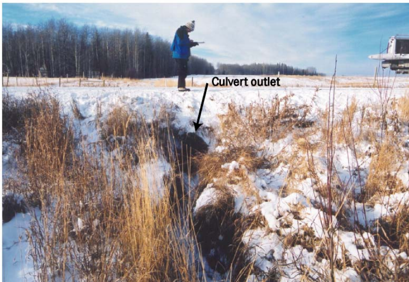
Plate 9. View of culvert outlet downstream of road. Note that channel is deeply entrenched immediately downstream of road (indicating that there is periodically scouring flows) (November 11/2002).
