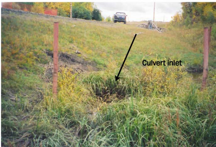
Plate 65. Culvert opening upstream of road. Note that grasses are providing stability to the soil relative to downstream of the road (September 20/2002).
