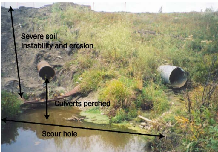
Plate 66. Dual Culverts downstream of road. Note extensive erosion and culvert perching (September 20/2002).
