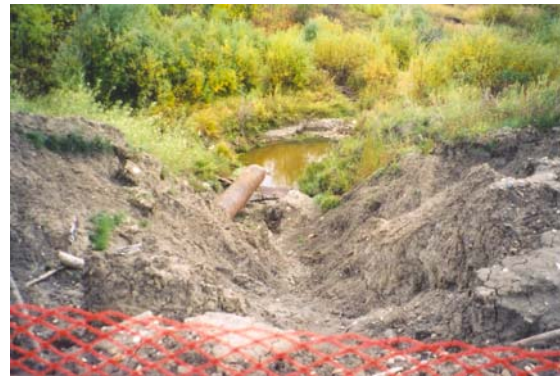
Unstable stream crossings in the Charlie Lake watershed are contributing sediment and sediment-bound nutrient loads to the lake and are thought to be accelerating lake in-filling and eutrophication rates.
