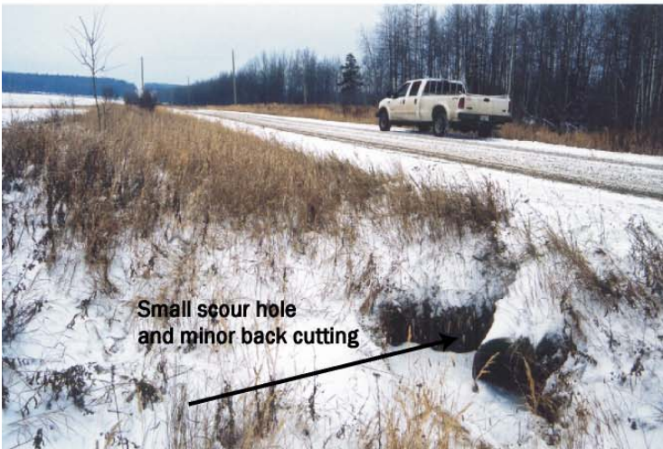
Plate 86. Culvert outlet downstream of road. Note slight backscouring (November 12/2002).
