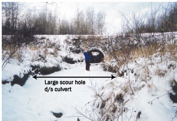
Plate 14. View of culvert outlet downstream of road. Note the large scour hole immediately downstream of the culvert (evidence of sediment movement) (November 11/2002).
