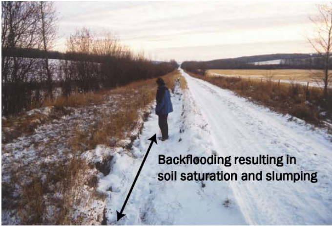
Plate 69. Back flooding upslope of road is resulting in soil saturation and slumping (November 12/2002).
