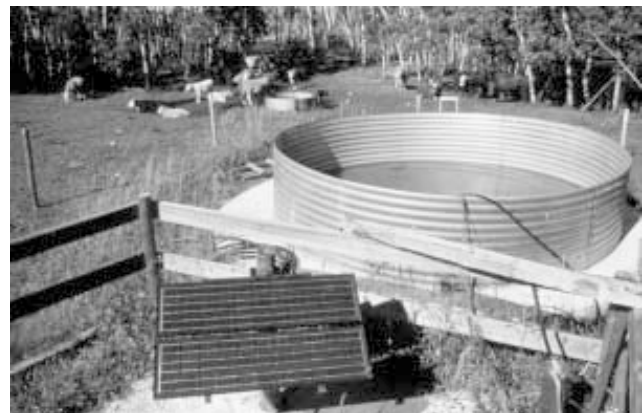
Figure 10. Solar powered well system
