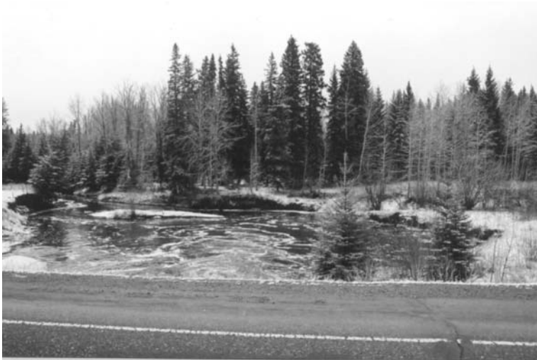
Massive scour hole downstream of a highway in the Dawson Creek, British Columbia area (Tupper Creek).
